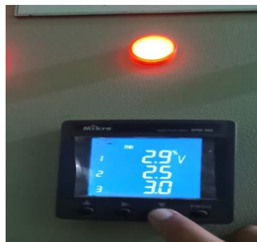
Figure 7 Digital power meter showing THDv (Total Harmonic Distortion Voltage) value in emergency room building.
