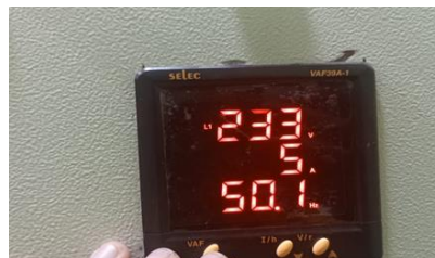
Figure 12 Digital Meter Shows the dimensions of L1, including voltage, current and frequency.
