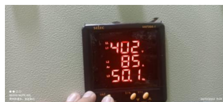
Figure 16 Digital meters display phase-to-phase or line-to-line magnitude. A digital meter reads 402 volts phase to phase
