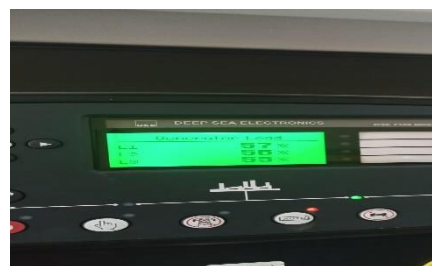
Figure 22. Documentation of Generator Load at L1, L2 and L3
