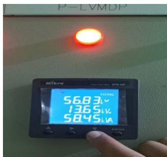
Figure 4 Electricity meter measuring kW, kV ar and kVa of the IGD . building
