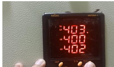
Figure 11 Digital meter in polyclinic building Displays voltage between lines.
