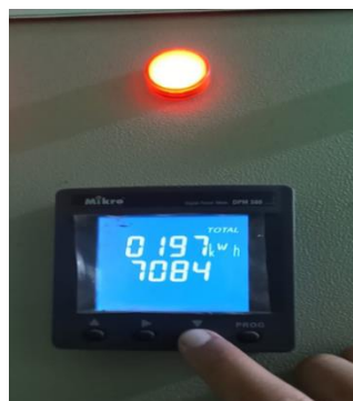
Figure 5 Emergency room building digital power meter measures active capacity.
