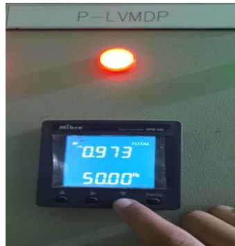
Figure 3 Digital power meters measure the power factor and frequency scales of an emergency room building.
