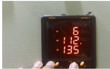
Figure 9 The digital clock in the polyclinic building shows the power.
