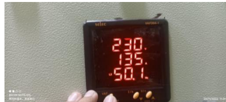
Figure 14 Digital Meter Shows L3 Magnitude Including Voltage, Current and Frequency
