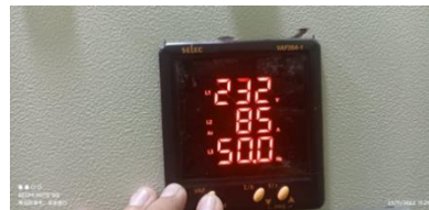
Figure 15 The digital meter shows the individual phase sizes and commutation averages or so-called averages of the distribution system.
