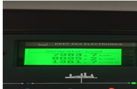
Figure 23. Generator load documentation on Generator Settings.
