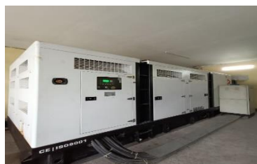
Figure 17. Documentation of the 800 kVa Generator Setting at Bhayangkara Hospital H.S. Samsoreri Mertojoso Surabaya
