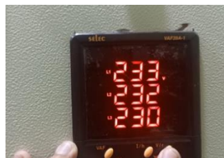
Figure 10 Digital meter in polyclinic building showing voltage on RS and T or L1, L2 and L3 lines.
